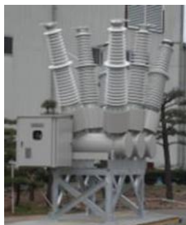
120 kV dead tank 1-break VCB
